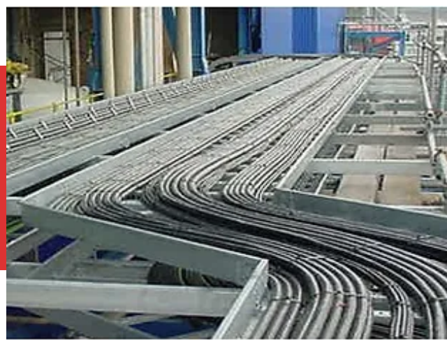
Indoor Fiber Cabling
