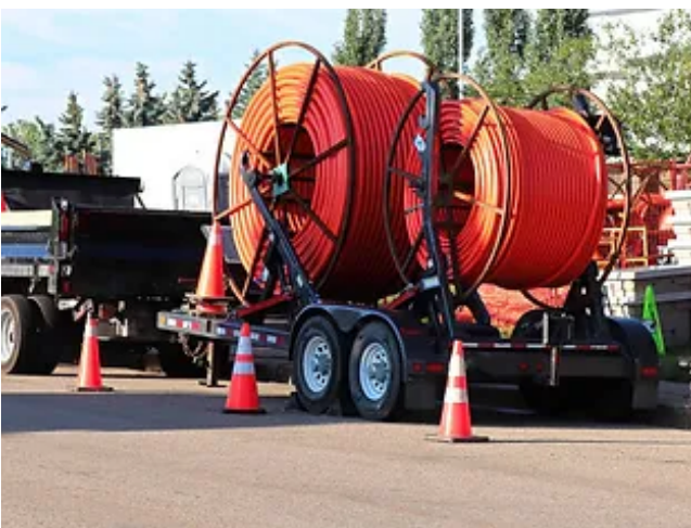
Outdoor Fiber Cabling
